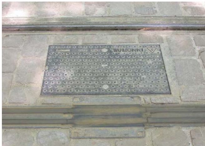
Fig. 16 - Power Box Installation
