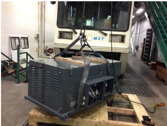
Figure 1 - Supercapacitor Energy Storage Unit being installed at Tri-Met in Portland, OR
