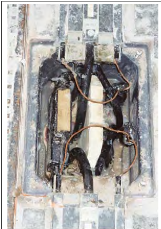
JUNCTION BOX INTERIOR
