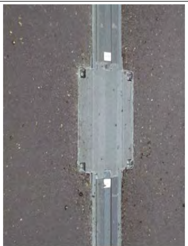
INSTALLED JUNCTION BOX
