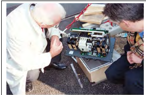
INTERIOR POWER RAIL CONTROL UNIT
