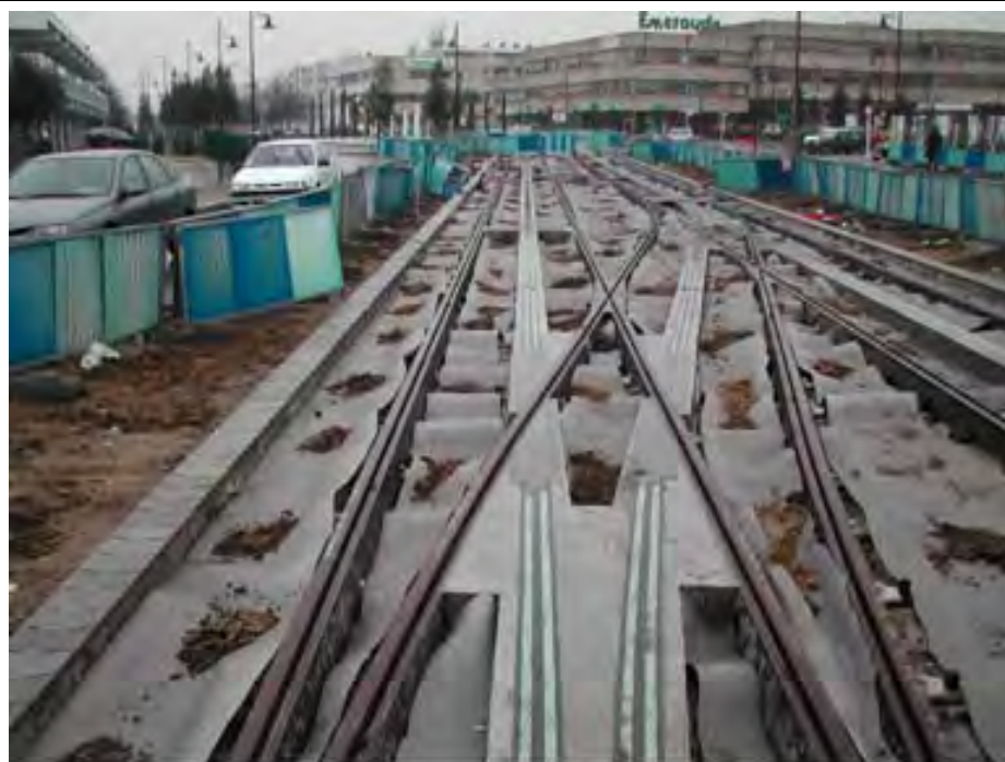
Crossing Special Trackwork
