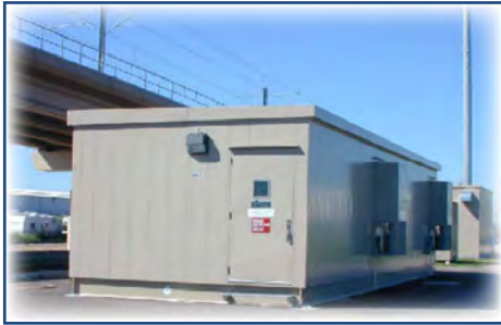
Traction power substation
