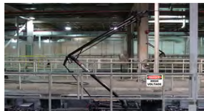
Exposed wires in shop
